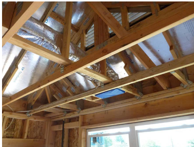
Figure 17: Below deck unfaced fiberglass batts and blown-in fiberglass on the ceiling floor.
